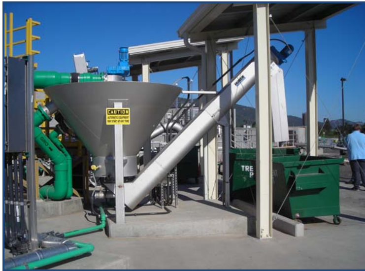
Figure 6: Huber Coanda Grit Washer System at Ukiah WWTP
