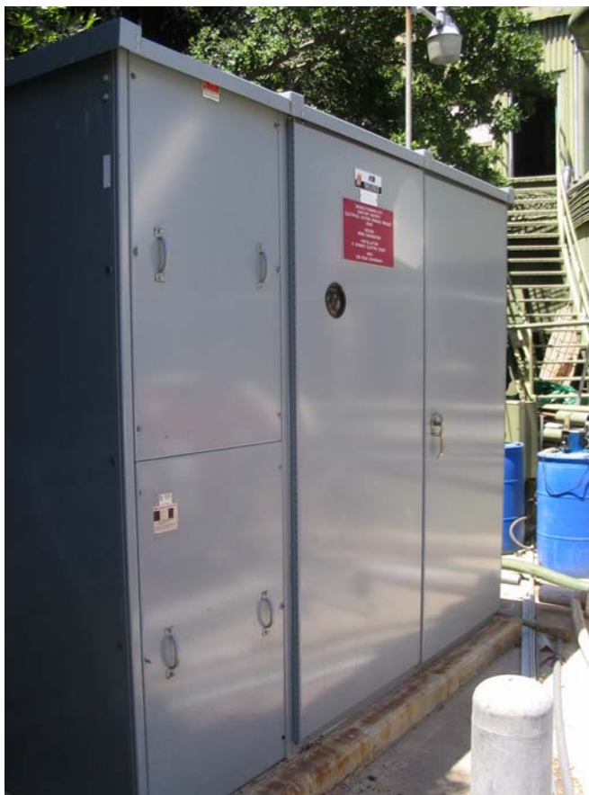
Figure 7.1.2 – Existing Main Service Switchboard (Section 1 and Section 2 ONLY. Third section on the right is a separate distribution panel fed by existing distribution panel H-2)
