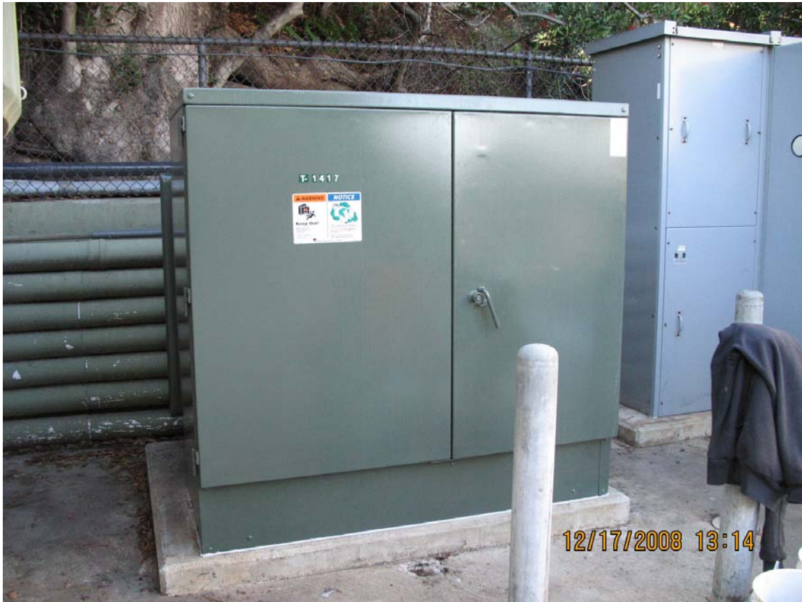
Figure 7.1.1 – PG&E Service Transformer T-1417
