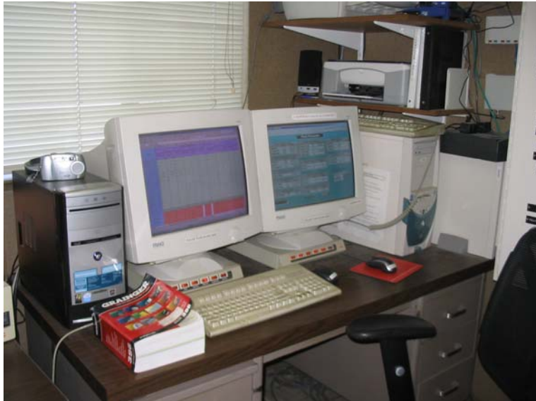
Figure 15.1.3 – SCADA Operator Interface Stations (Computers) in Operations Bldg.
