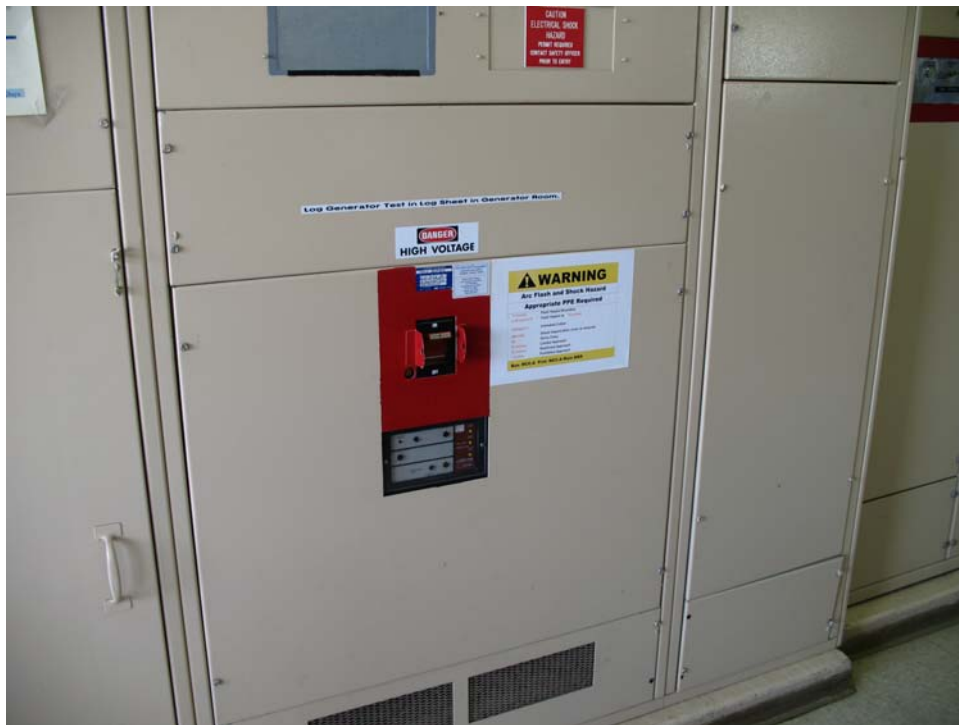
Figure 10.1 – Arc Flash Label on MCC
