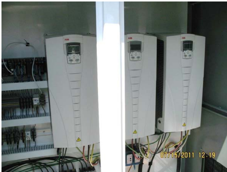
Photo 2 – Temporary Control Panel with three ABB VFDs
