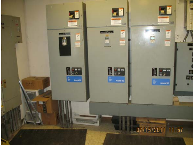
Photo 1 – Existing FFR VFDs
