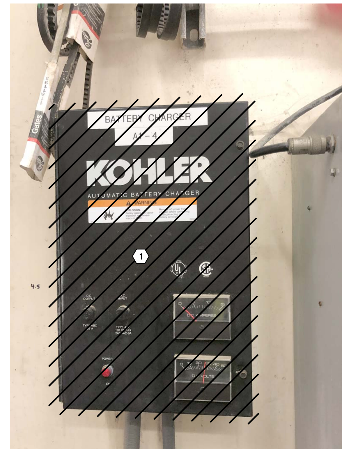
(A) EXISTING BATTERY CHARGER SCALE: NTS MAIN PLANT - GEN. BLDG
