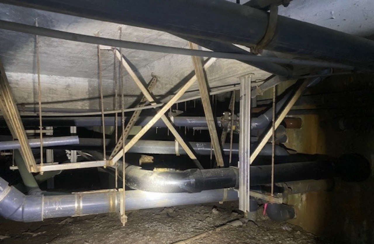
Piping Route is crowded.
