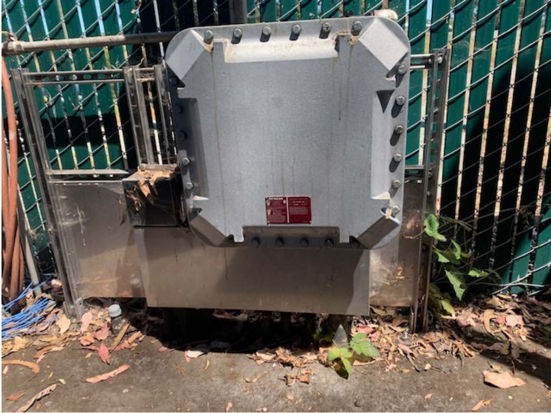
Stainless Steel shield/kick plate installed over air gap to protect exposed cables.
