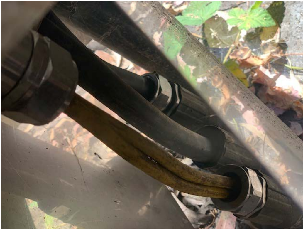
Cables exposed (air gap) to prevent gasses from reaching the termination cabinet.
