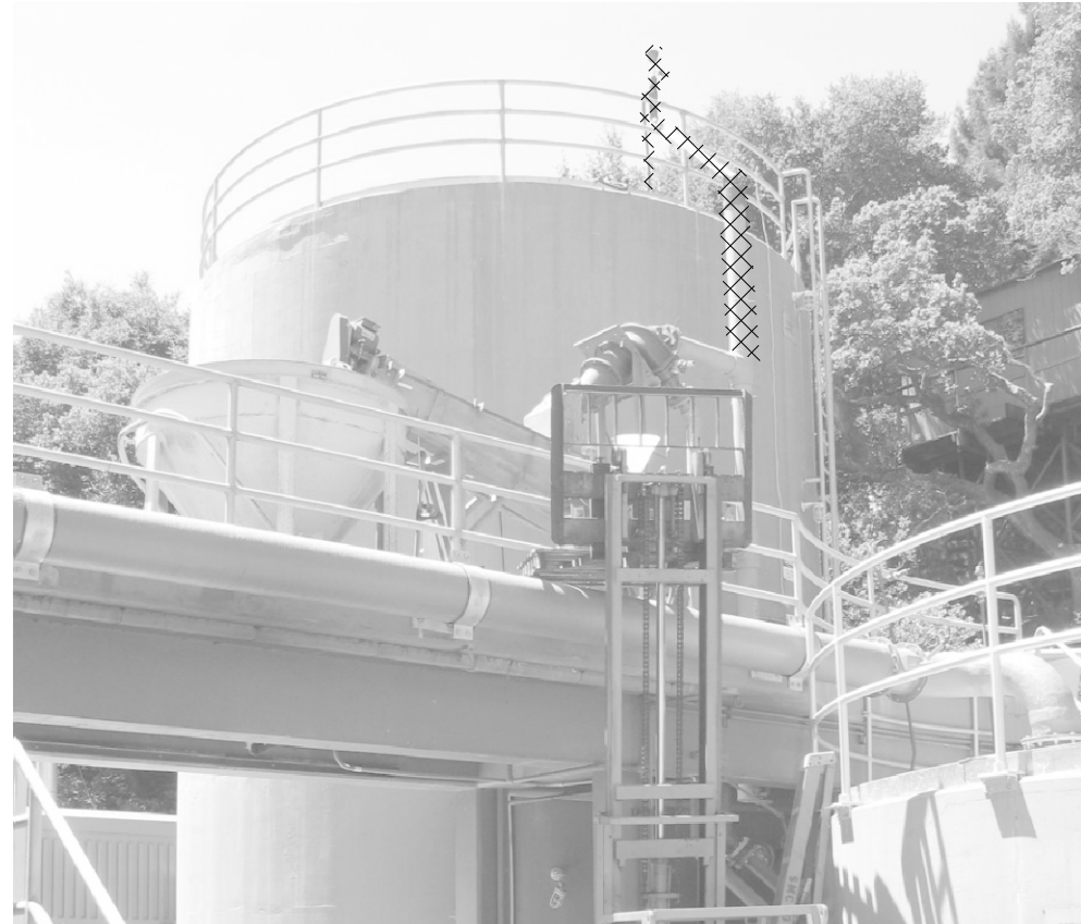
PHOTO P-3a (GRIT CLASSIFIER PIPING) NOT TO SCALE
