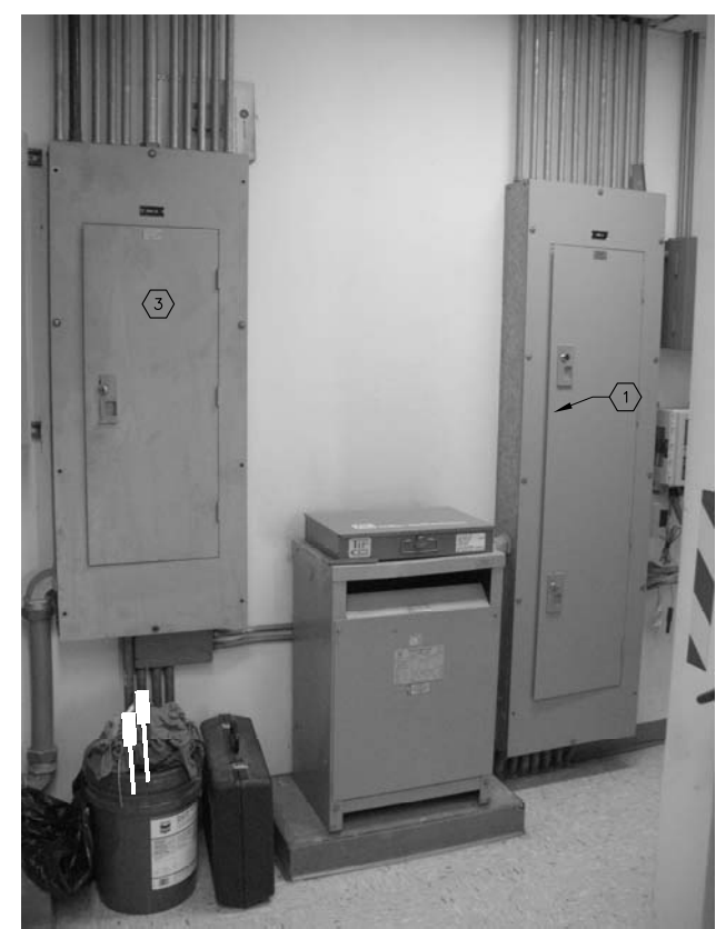
(A) EXISTING LIGHTING PANELBOARD "A" IN EXISTING CONTROL BUILDING SCALE: NTS
