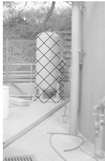
PHOTO (HYDROPNEUMATIC TANK) NOT TO SCALE P-1 M-1
