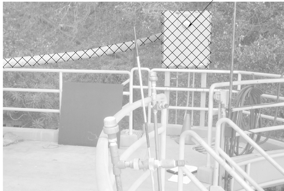
PHOTO (BUBBLER CONTROL PANEL) NOT TO SCALE P-5 M-1
