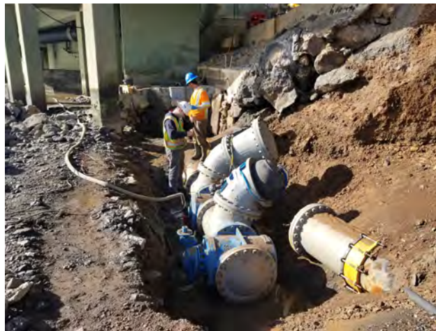
Beach Force Main Connection to Treatment Plant.
