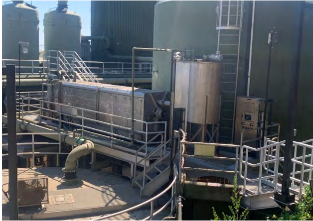
Existing screw press located on platform.
