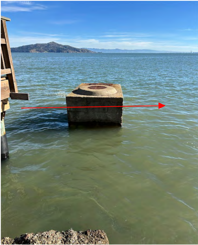
Photo 1: Inspection (pump station manhole); mainline runs in ocean through the manhole and follows direction in red arrow
