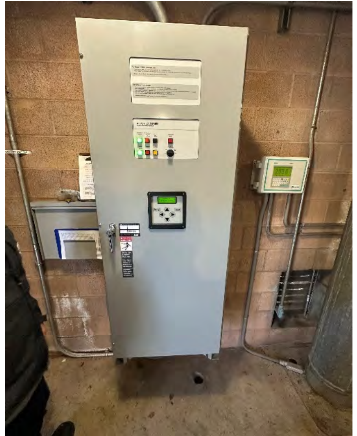
Photo 6: Inspection (pump station controls, view 2)
