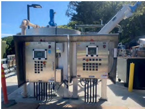
New Control Panels
