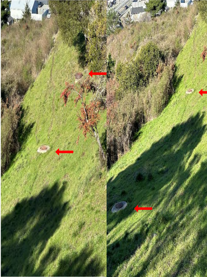
Photo 1: Inspection (easement mainline, view 1); crews The gravity sewer mainline runs along this sloped hillside and has no access for vehicle or heavy equipment; District field staff hand rod these sections of mainlines; all pipe has been lined recently to help reduce maintenance frequencies).
