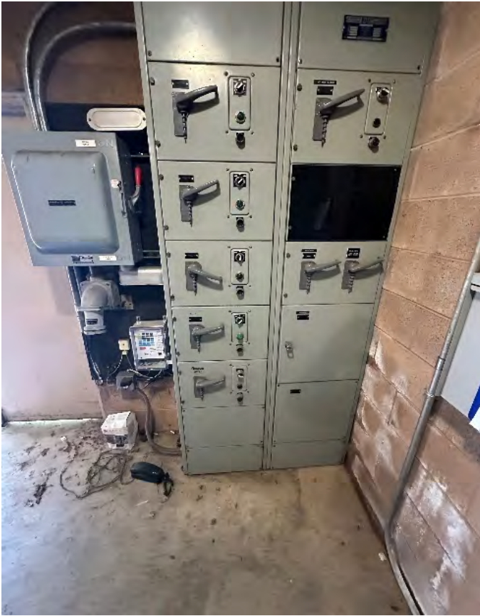
Photo 5: Inspection (pump station controls, view 1)
