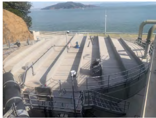
New odor control cover.
