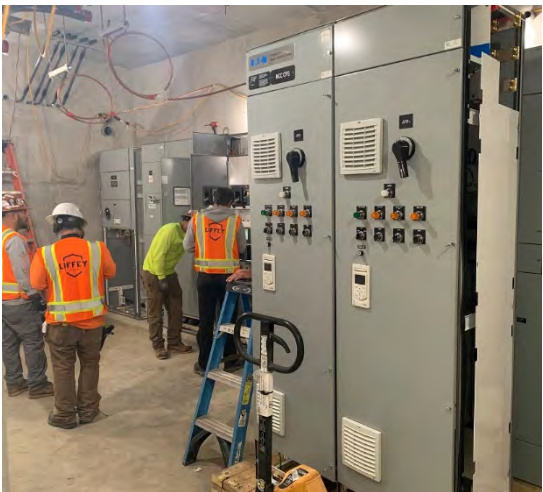
Underground controls building.
