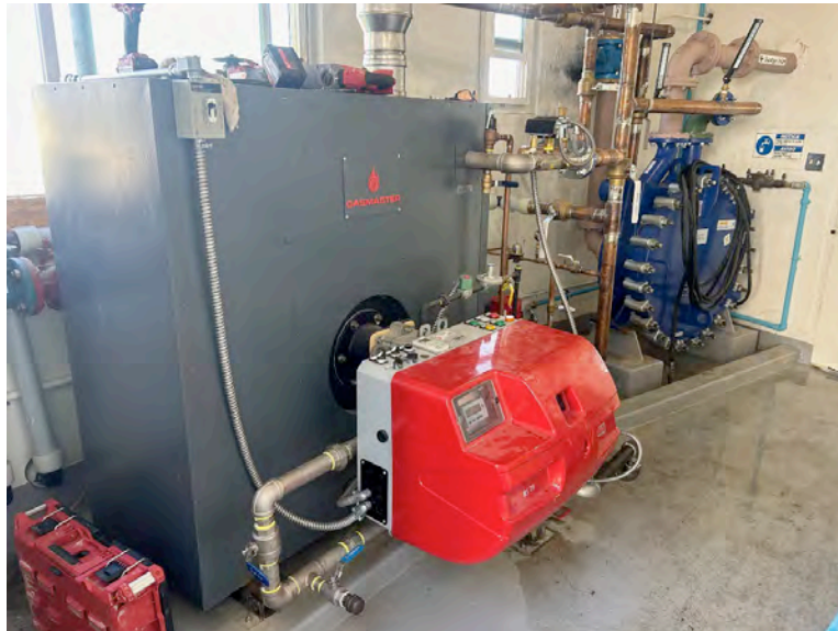
New boiler, heat exchanger and piping.
