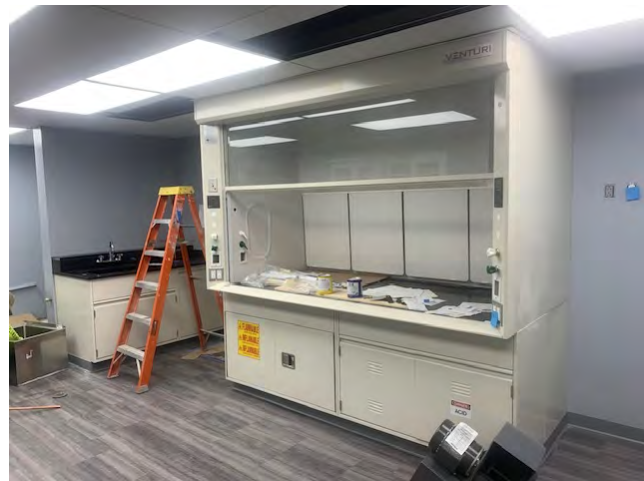
New vapor hood installation.
