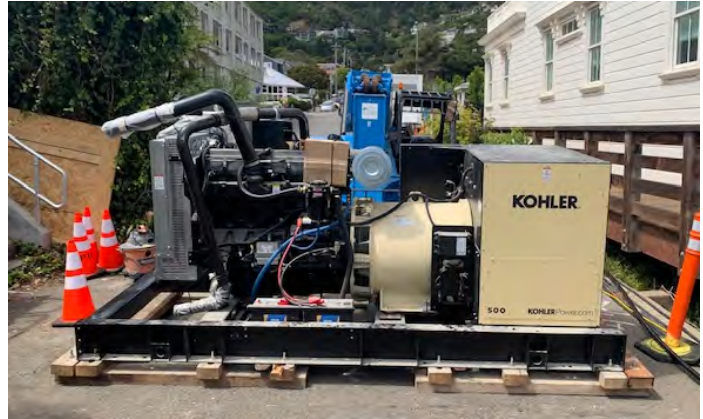
New Main St. Pump Station generator.
