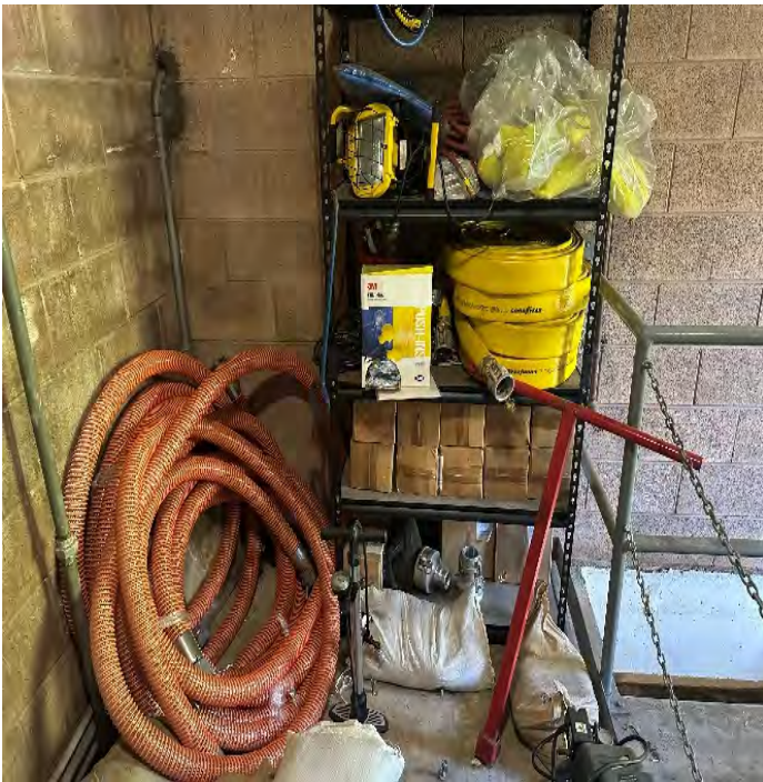
Photo 3: Inspection (pump station hoses stored onsite for emergency pumping including bypass equipment, view 1)
