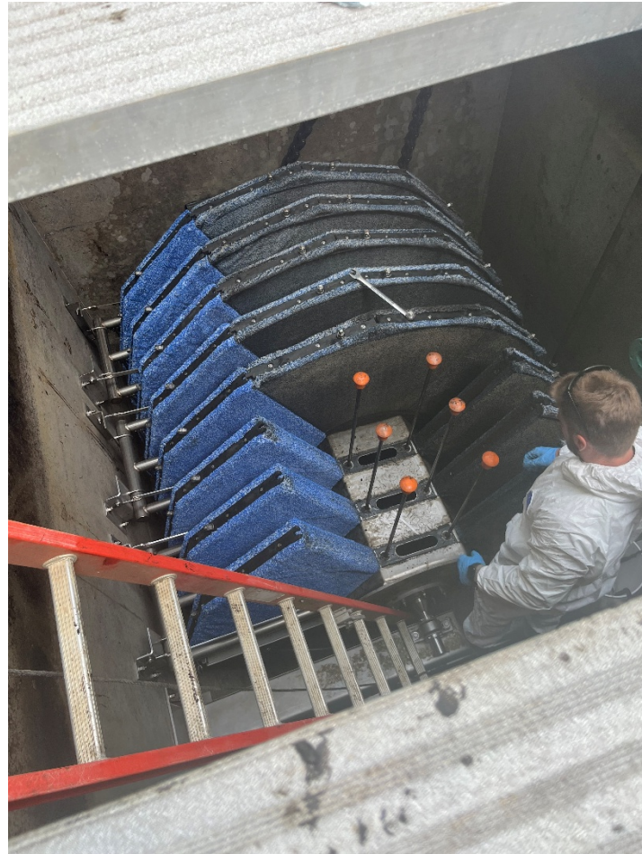
Removal Of Media
